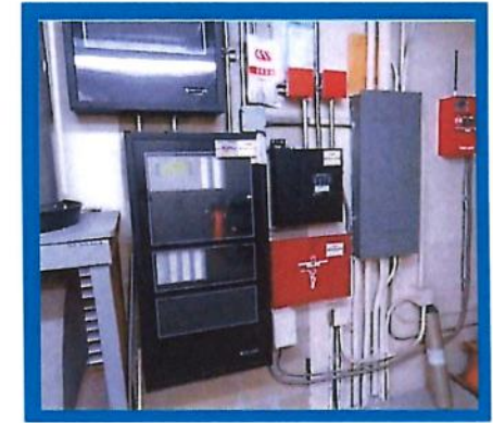
Life Safety Systems
