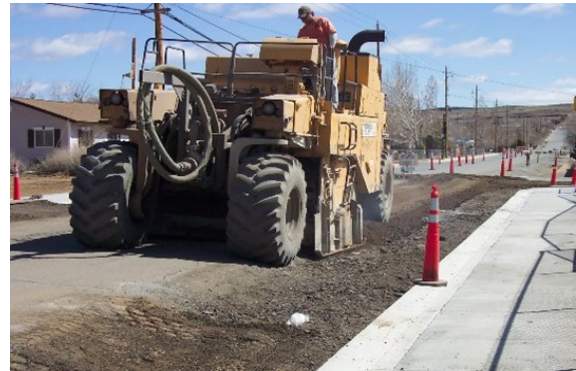
Pavement reconstruction costs about $3 to $4 per square foot in most residential settings.
