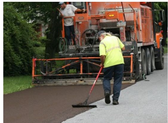
A pavement preservation treatment (such as this rapid-set slurry seal) costs about $0.20 to $0.30 per square foot in a residential setting.
